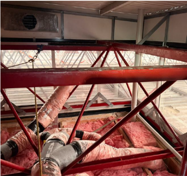
Photo 011 – Top and Bottom Chord and Diagonals (Amenities Building).
