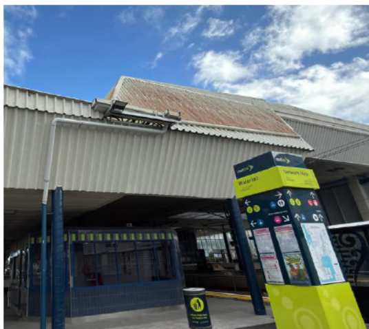
Photo 017 – Roof sheeting at Northern side of the station. Corrosion score 4.
