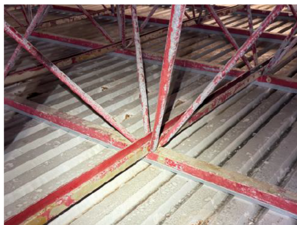
Photo 006 – Truss bottom chord. Corrosion score 1.
