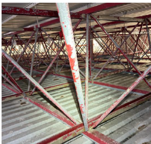
Photo 005 – Paint on truss diagonal has been stripped off.
