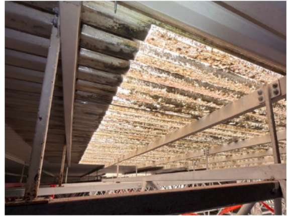
Photo 008 – Purlin Vertical Support Post. Corrosion score 3.
