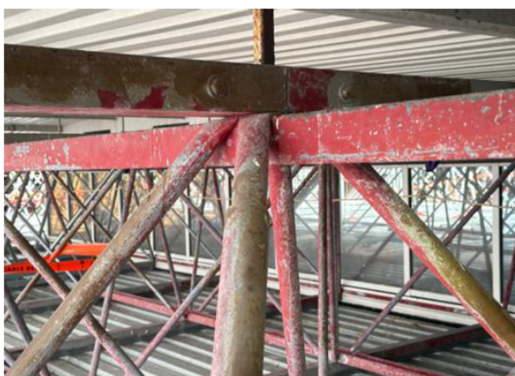
Photo 005 – Truss Top chord corrosion. Corrosion score 3.
