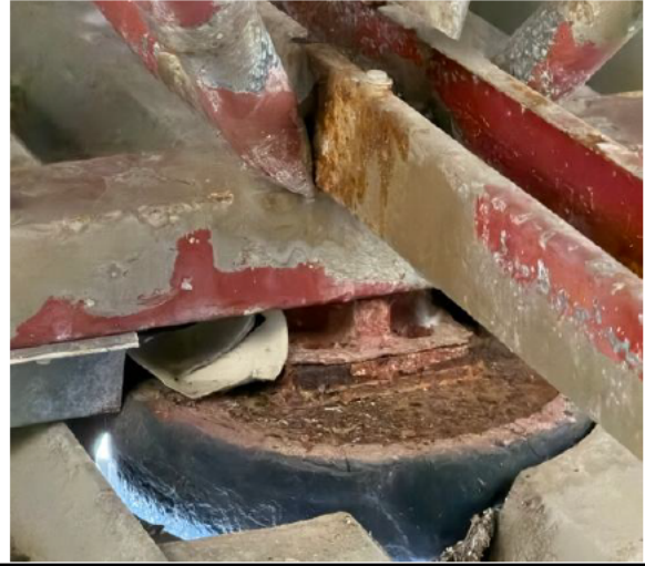
Photo 008 – Heavy corrosion between column and bottom chord. Corrosion score 4.
