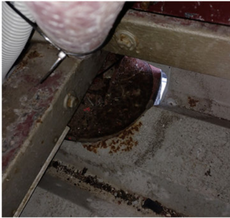
Plate between column and bottom chord corrosion score 4
