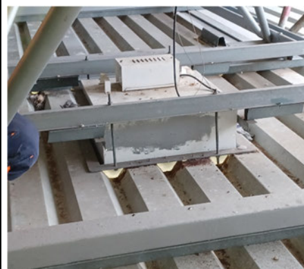
Corrosion spreading due to light fixings
