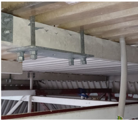
Purlin corrosion score 2
