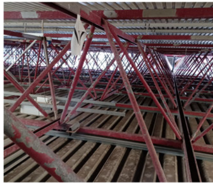
Diagonal corrosion score 2
