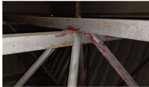
Truss top chord corrosion score 3
