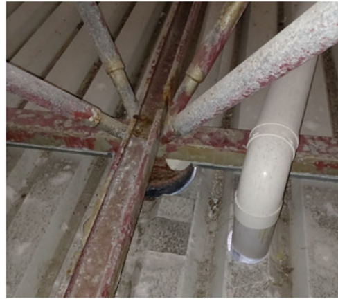
Plate between column and bottom chord corrosion score 4
