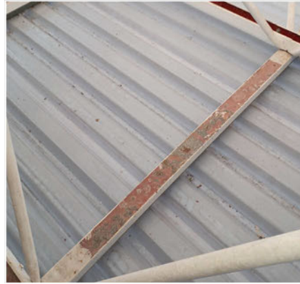
Bottom chord corrosion score 3
