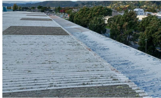
Orange Lyceum on lower roof corrosion score 4
