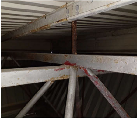
Purlin support corrosion score 4
