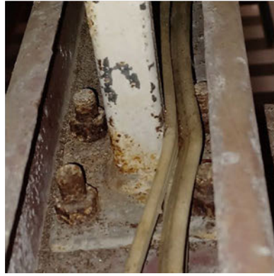
Purlin support corrosion score 3
