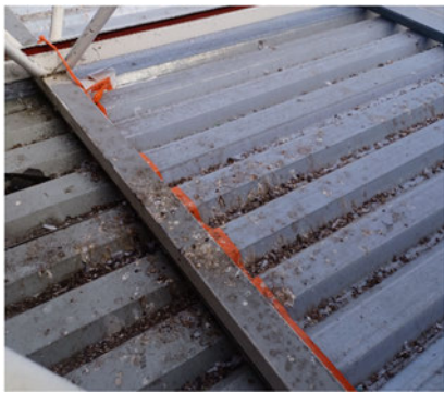
Accumulated Pigeon droppings
