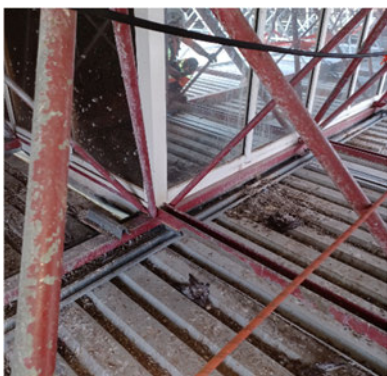
Accumulated Pigeon droppings
