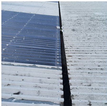
Internal Gutter corrosion score 2
