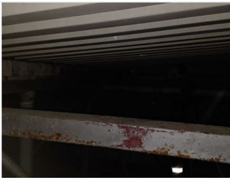
Truss top chord corrosion score 3
