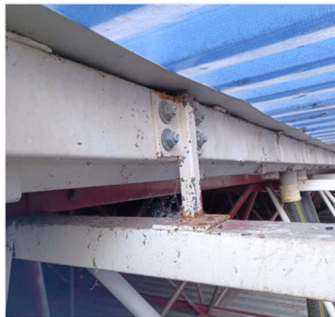
Purlin support corrosion score 4
