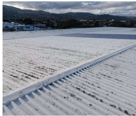
Ridge Capping corrosion score 2
