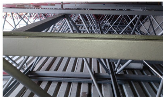
Diagonal corrosion score 1
