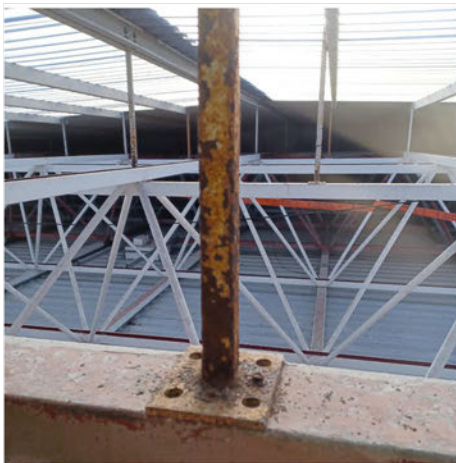
Purlin support corrosion score 4
