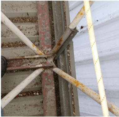
Diagonal corrosion score 3
