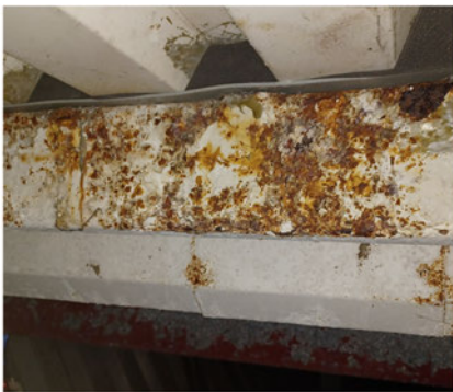
Purlin corrosion score 4
