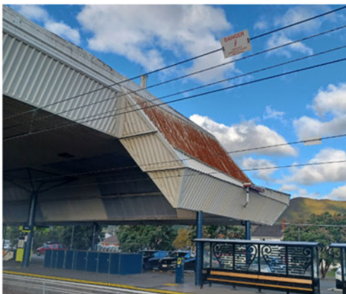
Orange Lyceum on lower roof corrosion score 4
