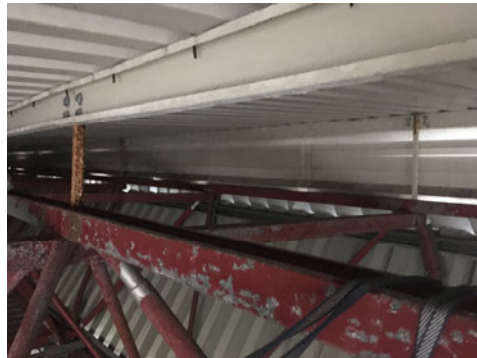
Purlin corrosion score 2
