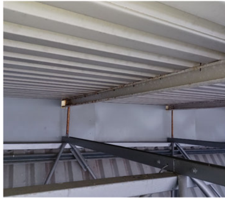
Purlin corrosion score 4
