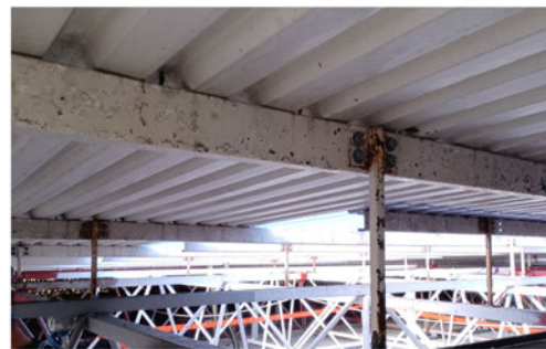
Purlin corrosion score 2
