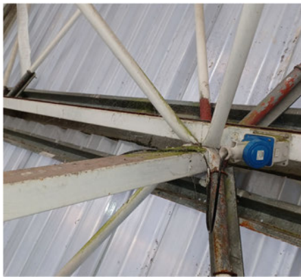
Diagonal corrosion score 3
