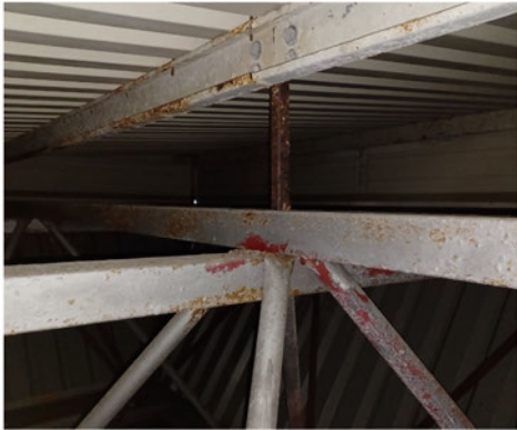
Purlin corrosion score 4
