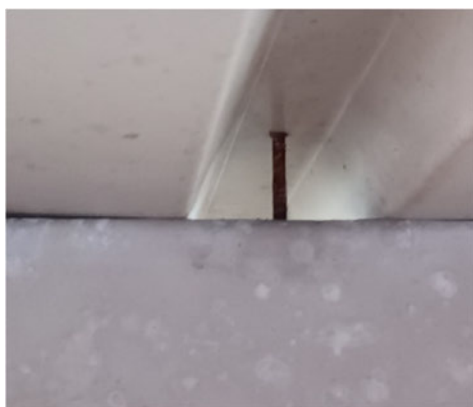
Corrosion at hold-down screws corrosion score 4
