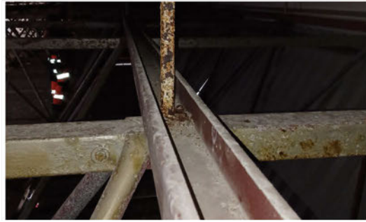
Truss top chord corrosion score 4
