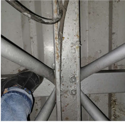
Bottom chord corrosion score 2
