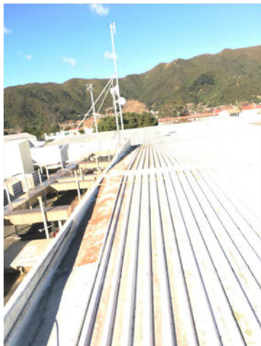
Roof seismic joint corrosion score 3
