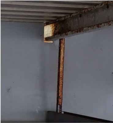
Purlin support corrosion score 4
