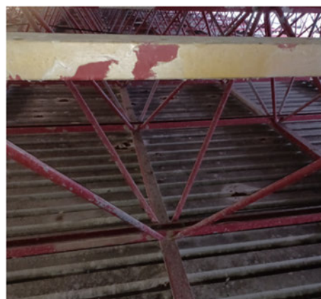
Corrosion at bottom roof sheeting corrosion score 4
