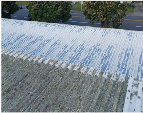
Roof Clearlite Panel corrosion score 3
