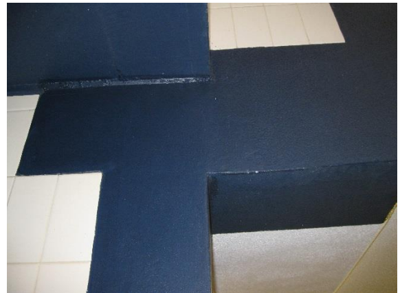
Photo 4 –Hair Line Cracks at the End of Tunnel
